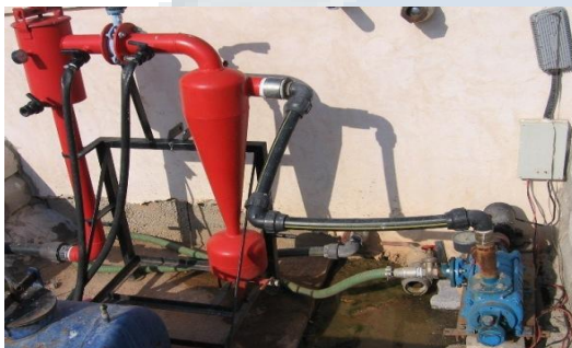
Fig. 7. BLDC-2, centrifugal pump and filters
