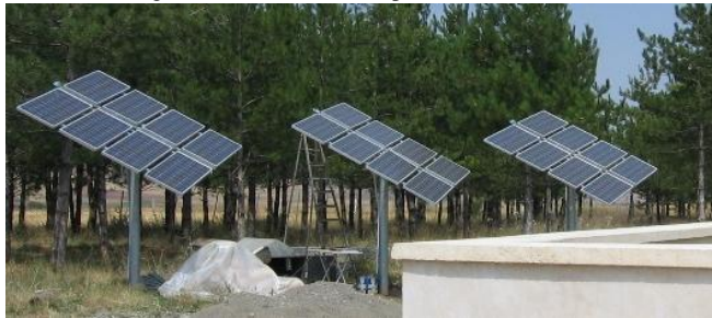
Fig. 6. Solar panels for BLDC-2 and water tank
